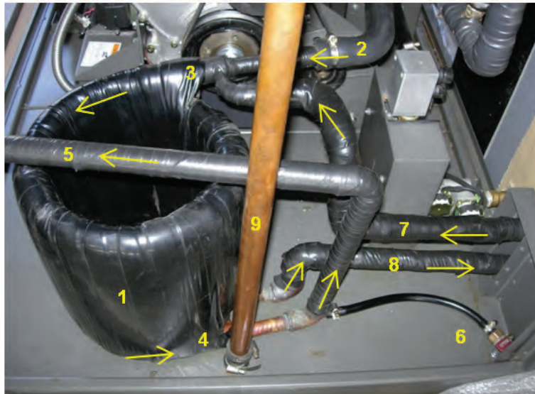
Fig. 7. Operating heat exchanger for heated water external system 1 – heat exchanger, 2 – coolant pipe from second heater on the exhaust pipe, 3 and 4 – start and end of parallel pipe system of engine cooling system (heat source) and external system (heat receiver), 5 – coolant pipe to engine radiator, 6 – valve for emptying engine cooling system, 7 – pipe with water to heat from external system, 8 – pipe with heated water to external system, 9 – overflow pipe carrying off water from the upper unit chamber, arrows – coolant and heated water circulation
