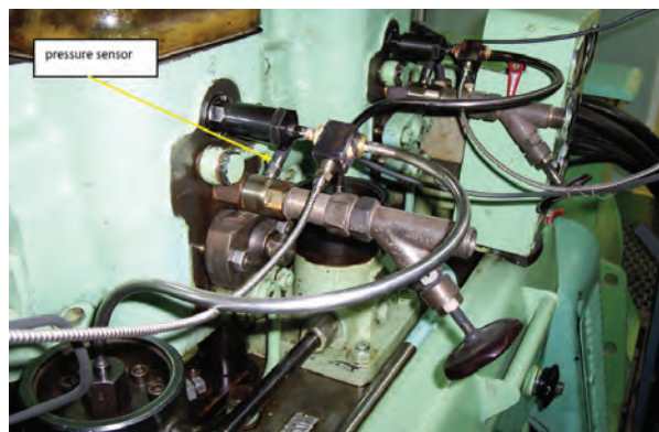
Fig. 1. Pressure sensor Kistler installed in indicator cock
