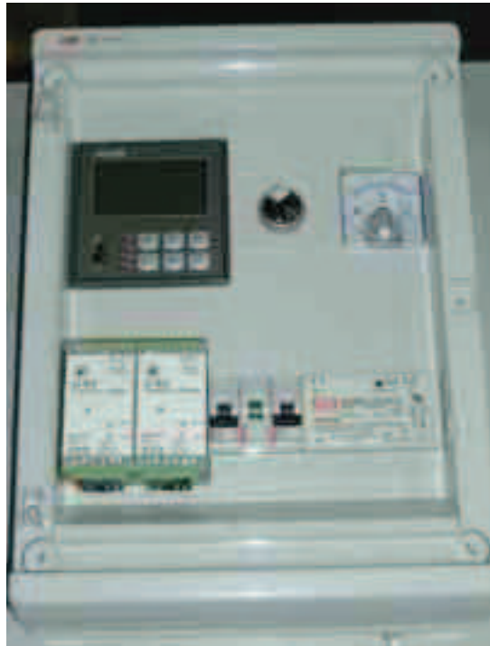
Fig. 2. Electrical power measuring and recording device
