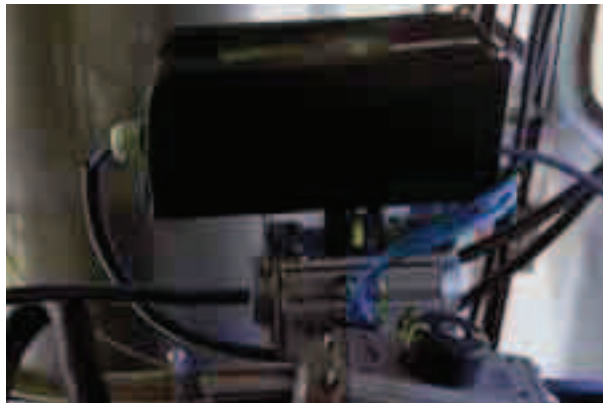
Fig. 4. A cold-water valve with a positioner
